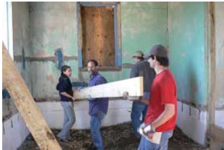
February 2008 New Orleans trip: Teamwork setting up floor joists. (Photo: Dan Stone)
